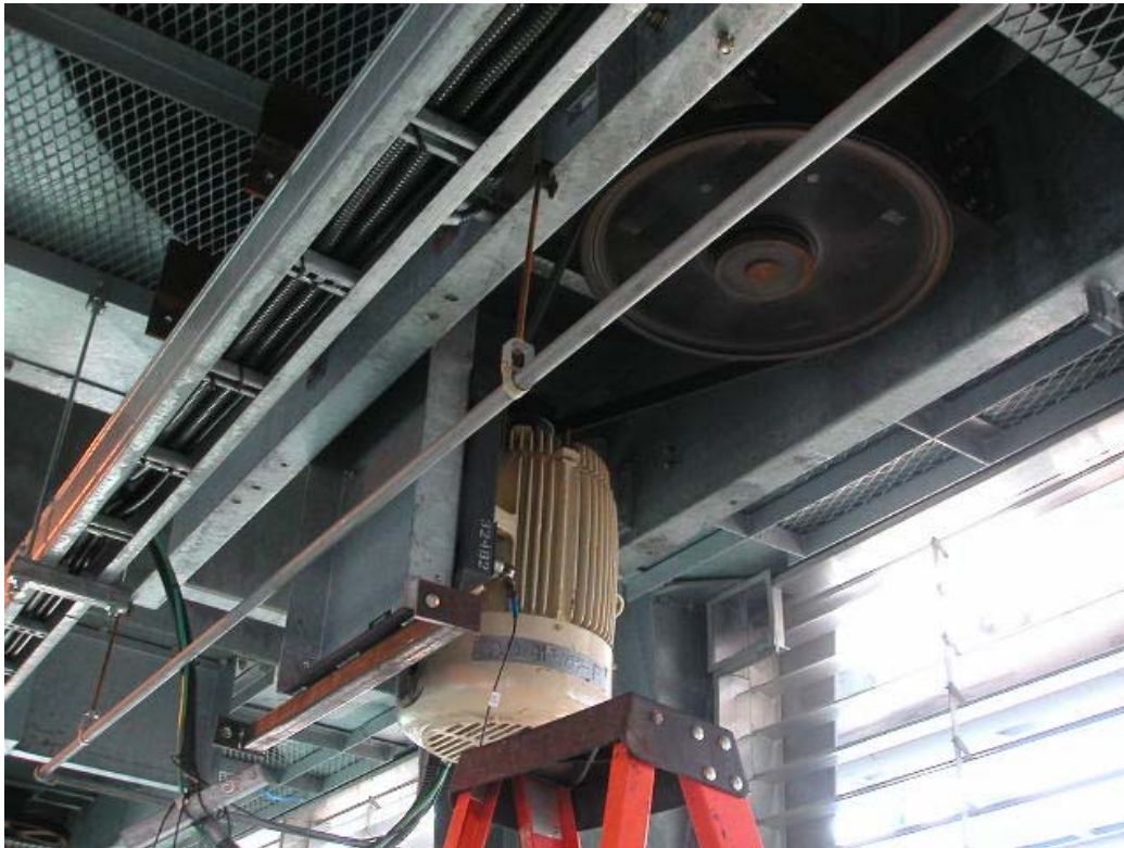
Figure 3.1. Motor, belt and driven sprocket on unmodified system
