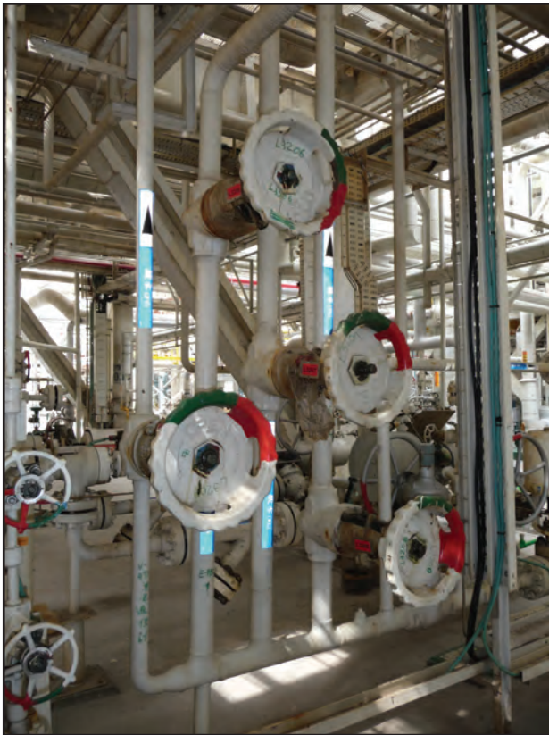
Photo 2. Triple redundant control system
