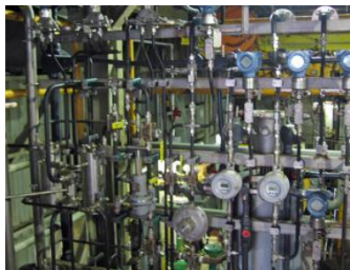
Dry Gas Seal Monitoring – a critical component of the system
