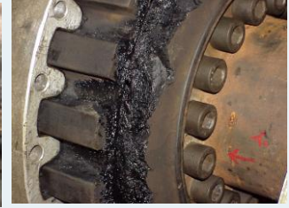
Melted rubber coupling
