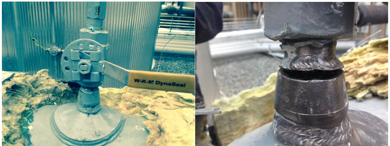
Figure 3. Original small bore attachment (left) and crack detail (right)
