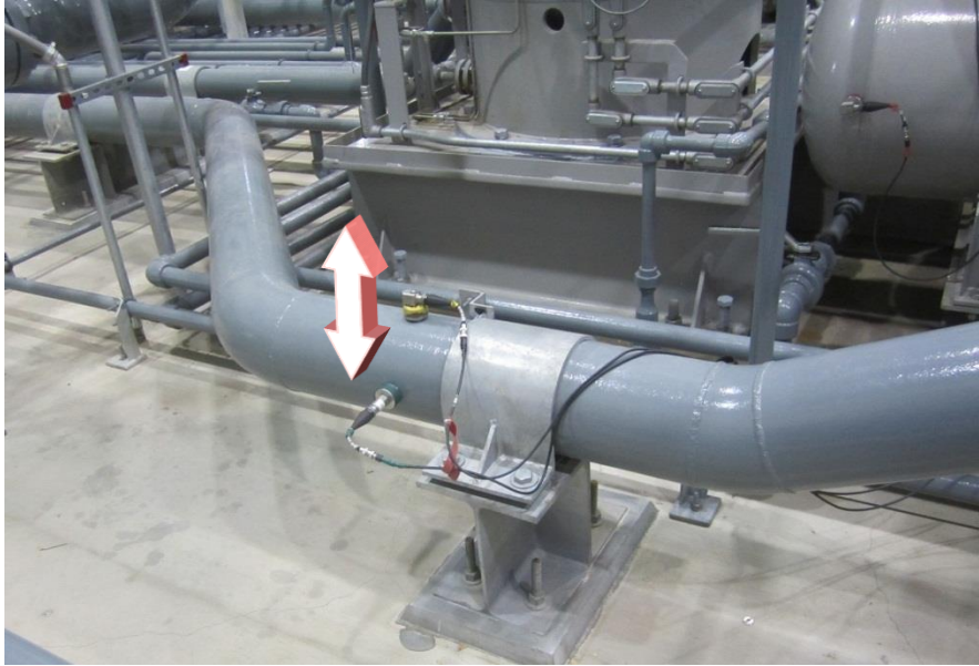
Figure 9. Discharge piping near discharge pulsation bottle
