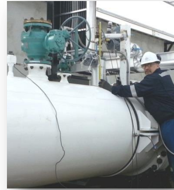
Figure 5: Piping Vibration Assessment (including small bore piping during normal and transient operations)
