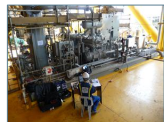
Figure 2: Field testing for vibration on skid and structural beams
