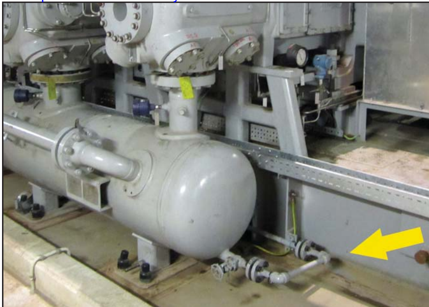
A drain line (see arrow) on a discharged bottle failed twice due to high vibration, causing safety hazards and requiring repairs at a refinery.
