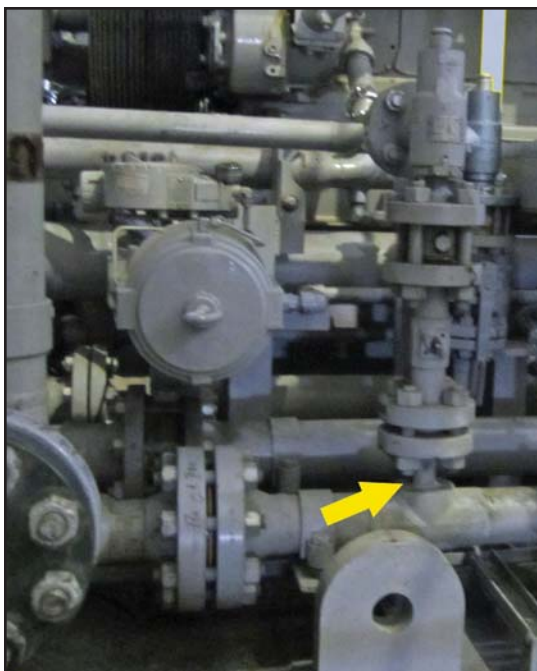
At a compressor station, this small-bore piping (SBP) (see arrow) failed at the connection to the main piping, causing a gas release and fire.
