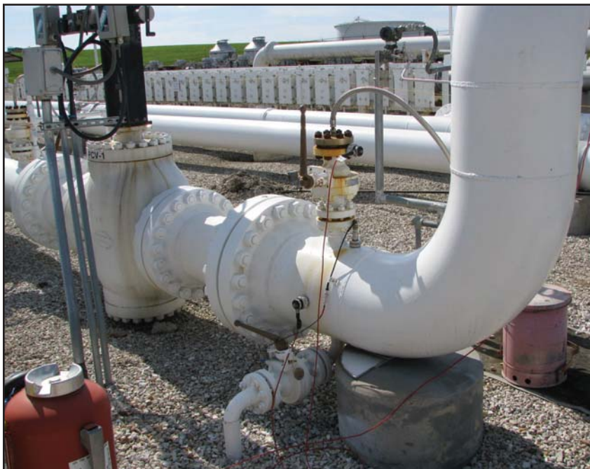
An oil pipeline is wired for a SBP analysis.
