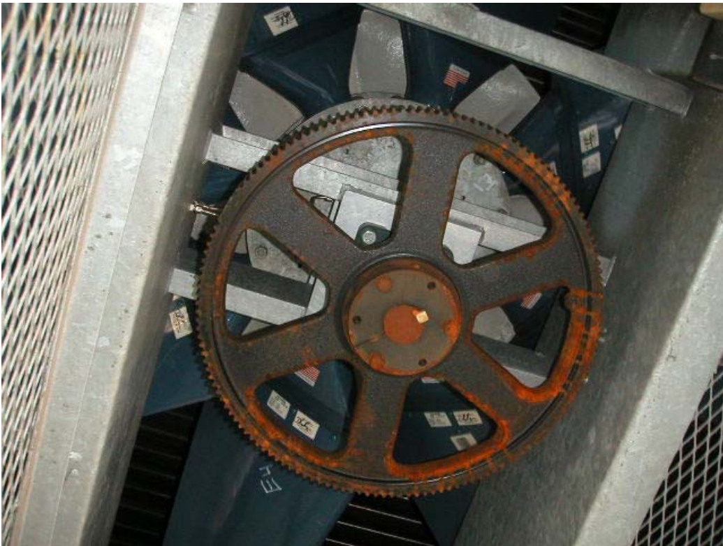
Photograph 2: Fan and driven sprocket viewed from below
