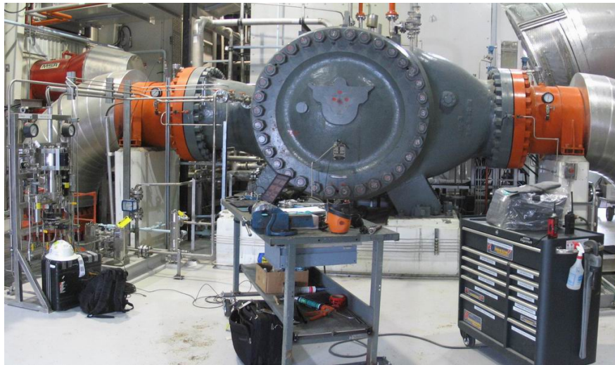
Figure 1: One of three centrifugal compressors that experienced vibration problems due to mechanical and acoustical resonance
