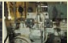
Optimized equipment to improve plant throughput and reliability.
