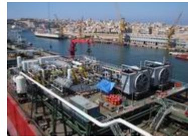
FPSO design for two, 3500 HP compressor units constructed in Malta
