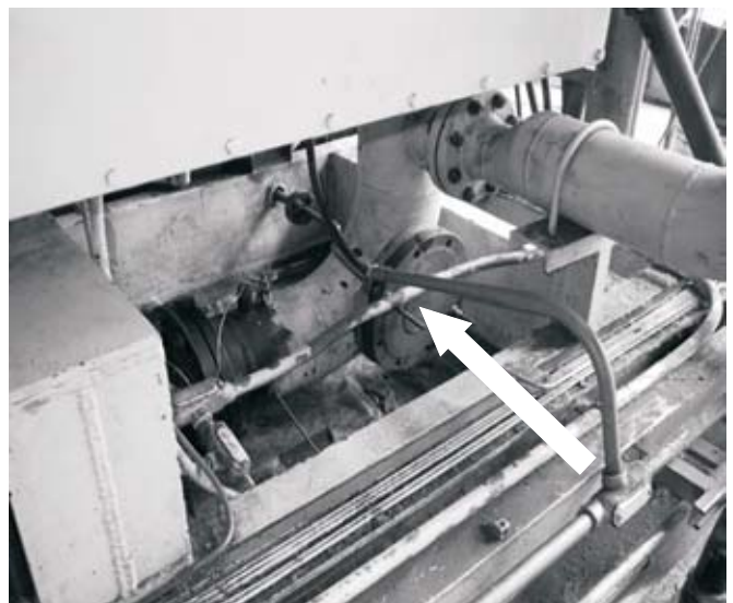
Figure 6 Discharge line de-tuning weight located at lower elbow before D118
