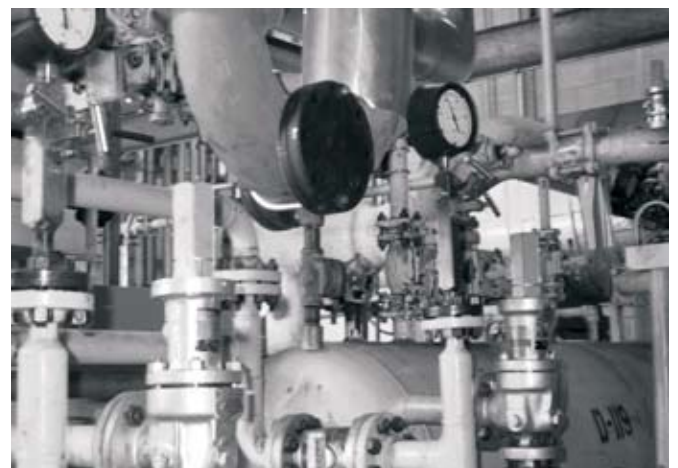
Figure 3 Discharge piping from vessel D118 with de-tuning weights secured
