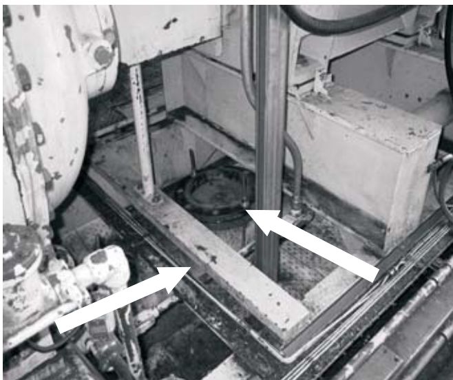
Figure 5 Discharge line de-tuning weight located under compressor/motor coupling
