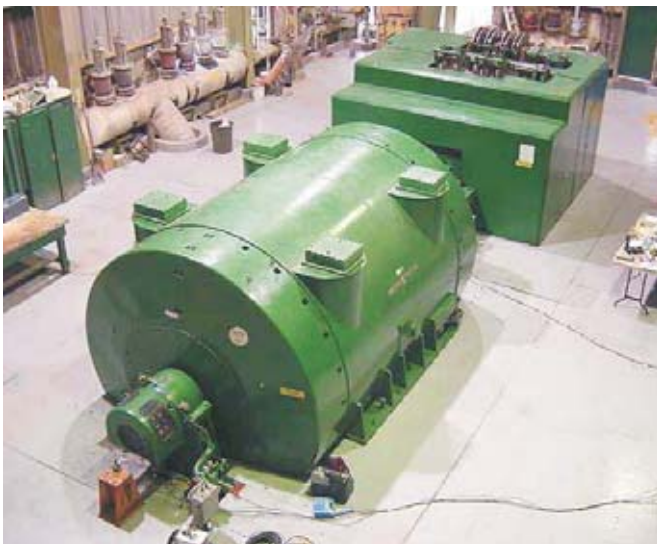
Figure 1. Overall view of the turbo generator.
