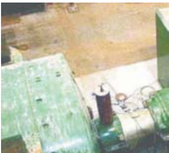
Figure 6. Tuned mass damper installed on inboard generator pedestal in 2001.
