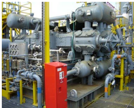
Figure 4: Example of Reciprocating Compressor on FPSO. Dynamic analysis of compressor forces on FPSO structure requires coordination between Machinery Consultant, Packager, and Engineering Consultant.
