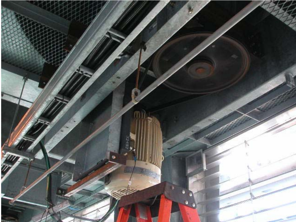
Photograph 1: Motor, belt and driven sprocket on unmodified system
