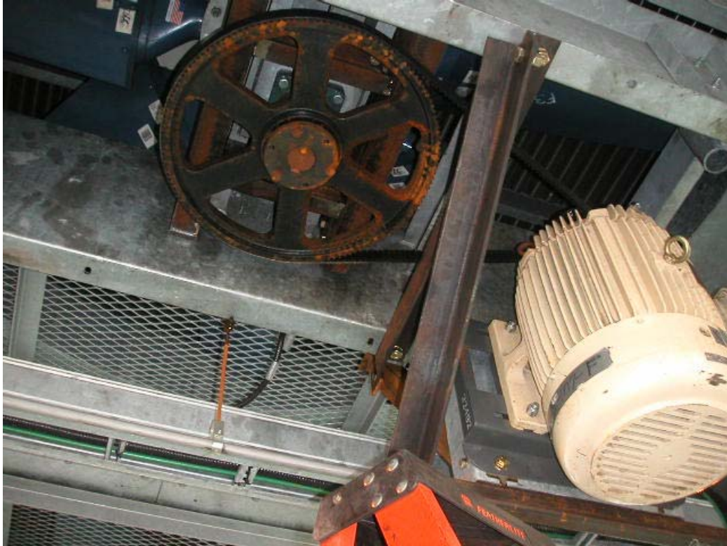
Photograph 3: The photograph above shows one side of the bracing. The stiffening was primarily in the north-south direction.
